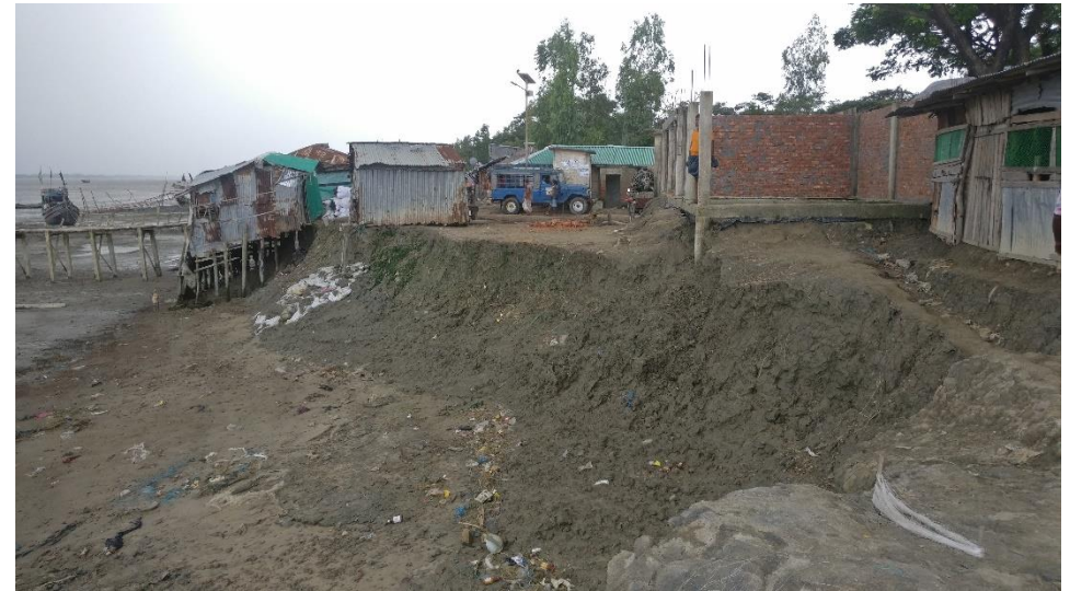
Figure 23: Broken part of the embankment in akbar balir ghat
