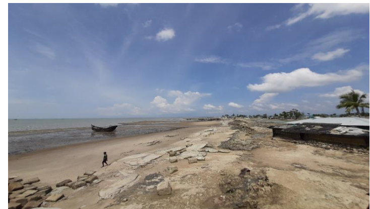
Figure 25: Broken part of the embankment in ward 1 and cluster villages are fully exposed
