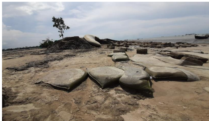
Figure 24: Broken part of the embankment in ward 1
