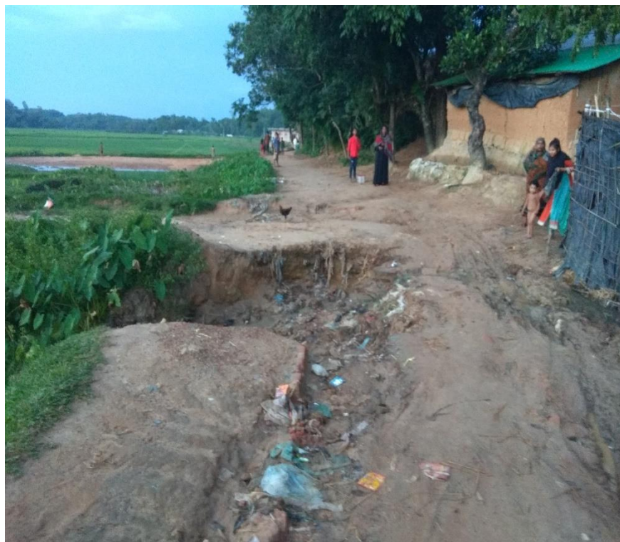
Figure 12: Flat soiling road from Kasarimora school to Main road, in ward no 1
