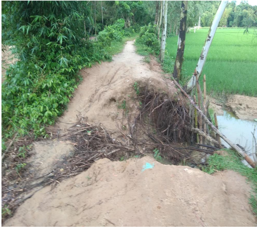
Figure 11: road in ward no 1
